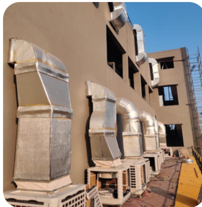
Air Cooling Work – Specialized cooling system for large-scale facilities.
